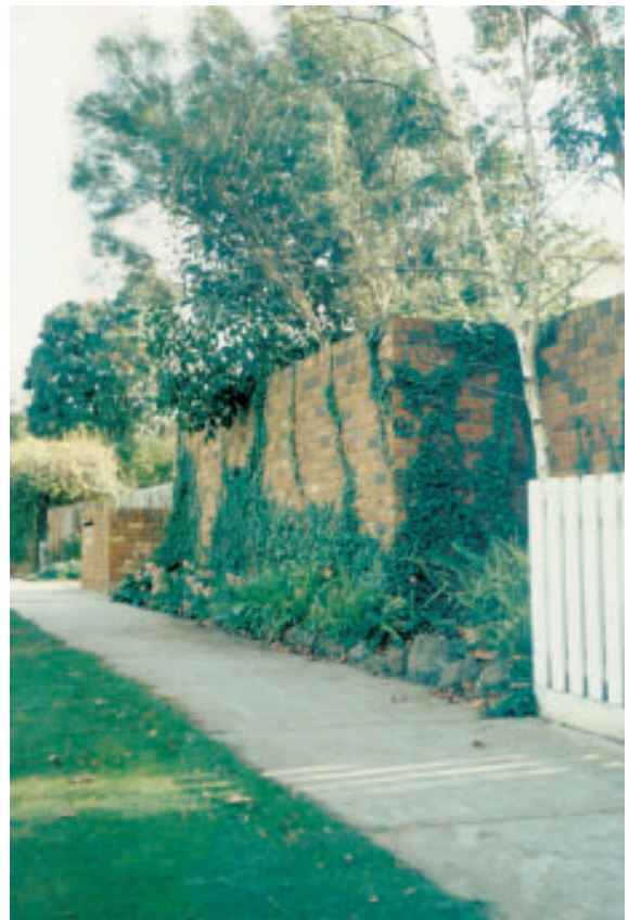
Part of the wall has been stepped back to permit planting. Creepers have also been used to enhance the appearance and soften the hard lines of brickwork
