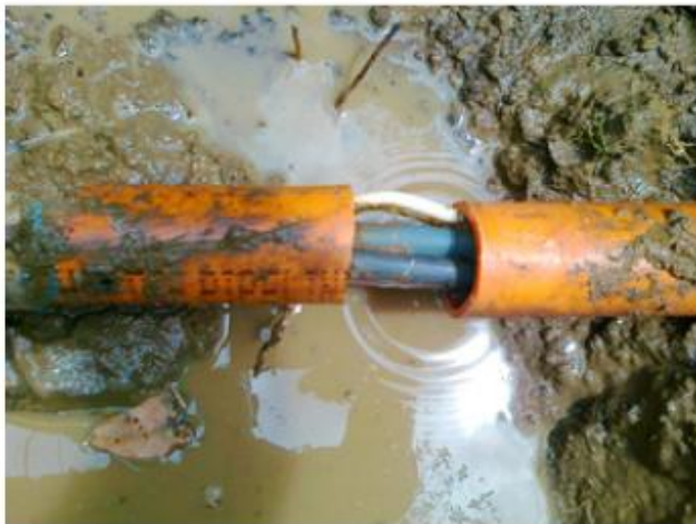
Photo 1: Separate circuits within the same conduit.
