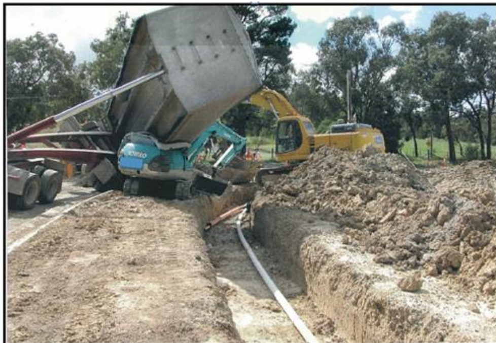
An example of what can occur if a trailer overturns. Fortunately the operator of the excavator was not in the machine at the time
