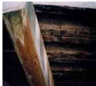
Fig 5 - Longitudinal crack at corners of crosshead associated with corrosion of steel reinforcement
