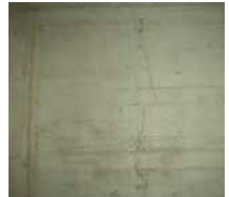
Fig 4 - Drying shrinkage cracking
