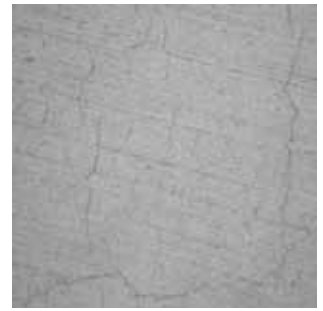
Fig 2 - Plastic shrinkage cracks
