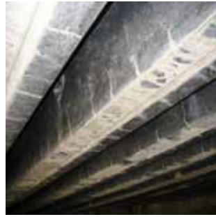
Fig 1 - Flexural cracks that self sealed through autogenous healing
