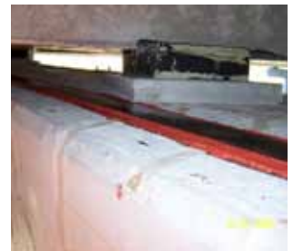
Fig 6 - Active or live cracks sealed with an appropriate flexible sealant
