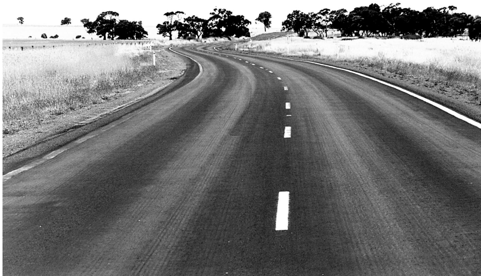
Figure 1: LH wheelpaths flushed, this would be indicated by low textures in RAS outputs.
