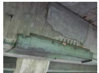
Fig 6 - Saw cutting of perimeter of repair area, application of steel primer, formwork in place, and repair with free flowing micro concrete in formwork
