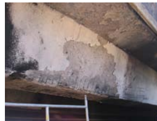
Fig 3 - Concrete surface skin detached from upper part of beam
