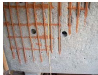
Fig 5 - Preparation to sound and dense concrete, exposure and protection of steel, shows coring holes
