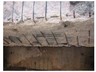
Fig 2 - Explosive spalling, pink tint, exposure of steel ligatures, main corner bars and pre-stressing tendons. Temperature above 300°C
