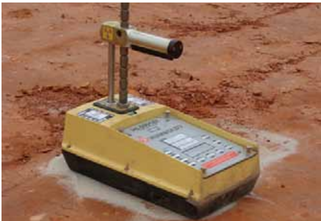
Figure 6 NDG soil meter on earthworks test site with test probe at test depth of 175 mm
