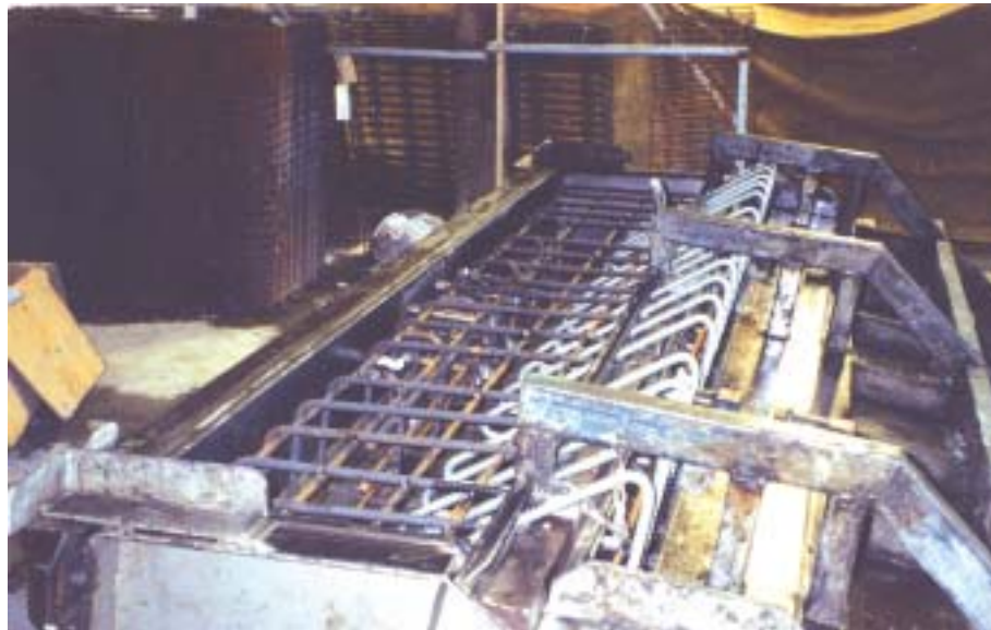
Figure 7.1 Surveillance reports may include photographs or comment on items such as formwork preparation ready for casting a bridge parapet.
