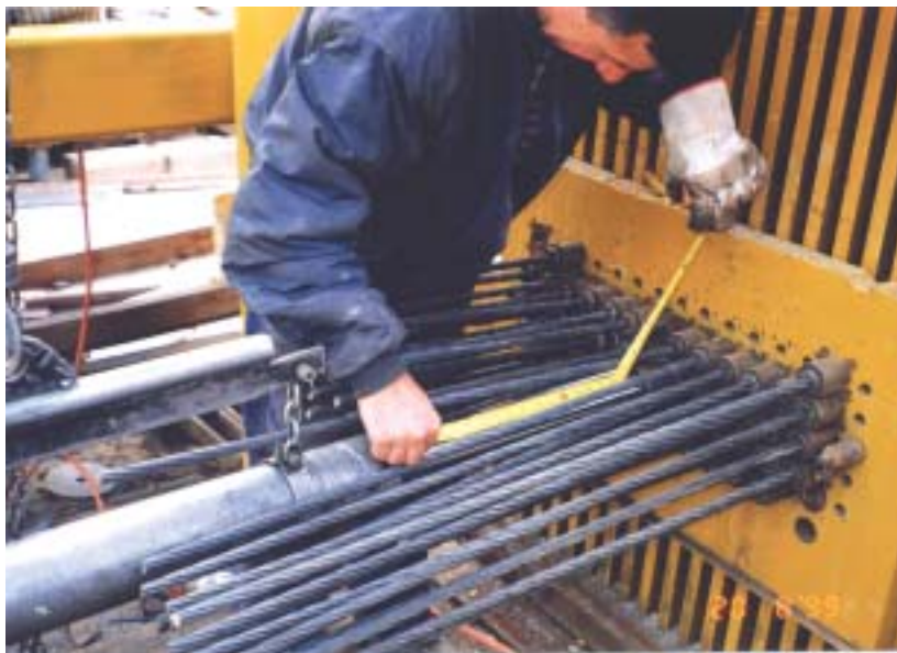
Figure 6.1 A Surveillance Officer must ascertain that specified testing is carried out, such as measuring elongation of tendons during stressing operations, pictured here
